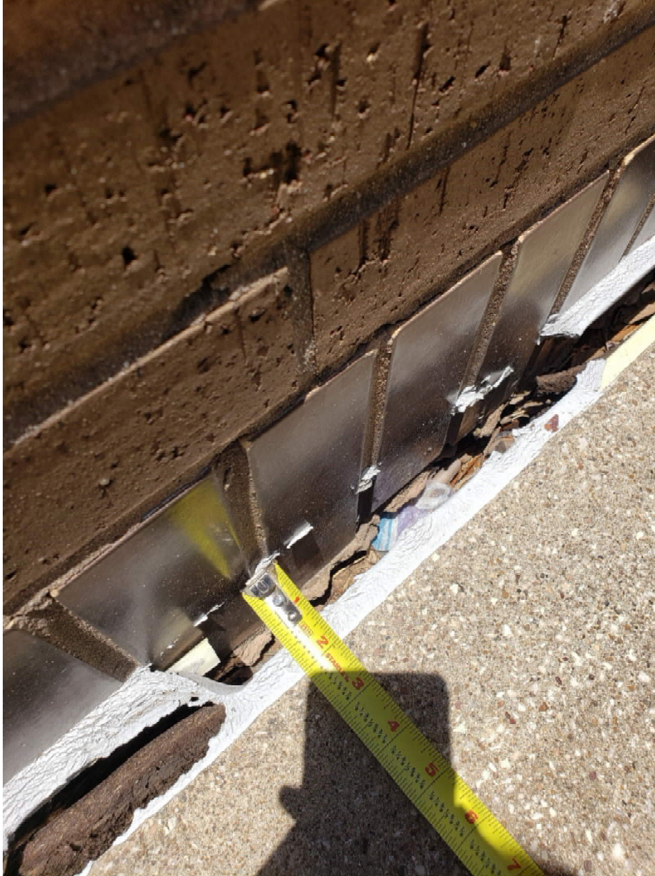
Description: 2-Inch Horizontal Movement between Exterior Cladding and Adjacent Paving
