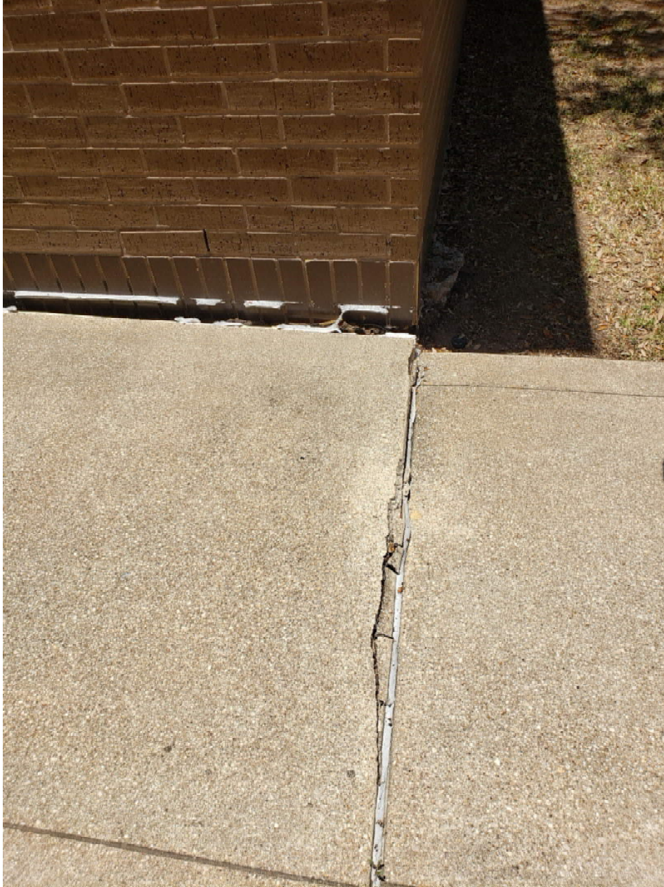
Description: Cracks in Adjacent Paving
