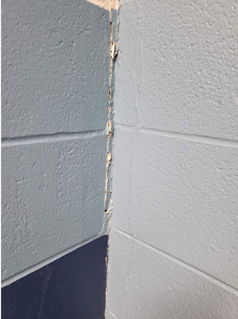
Description: Cracks in Non-Load Bearing CMU Walls in Music Hall on Level 1
