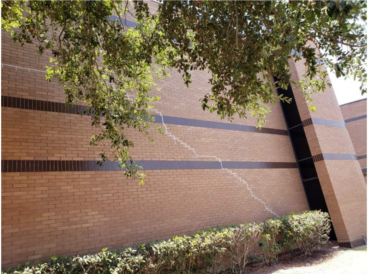
Description: Cracks Exterior Brick Cladding
